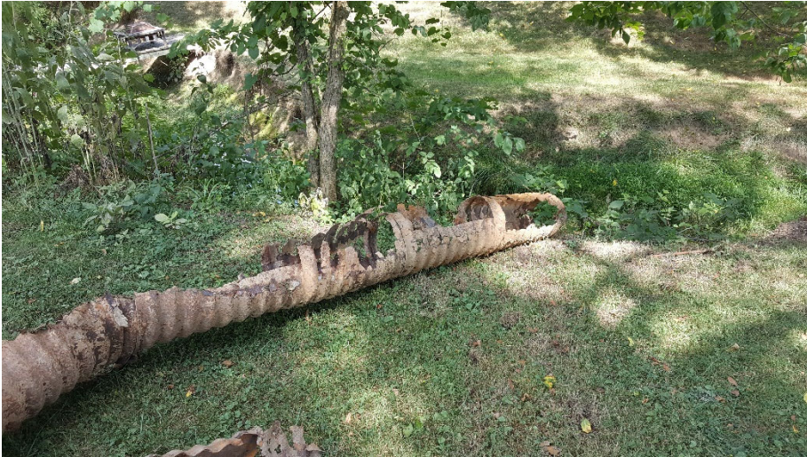
Deteriorated metal pipe removed from Judith Drive
